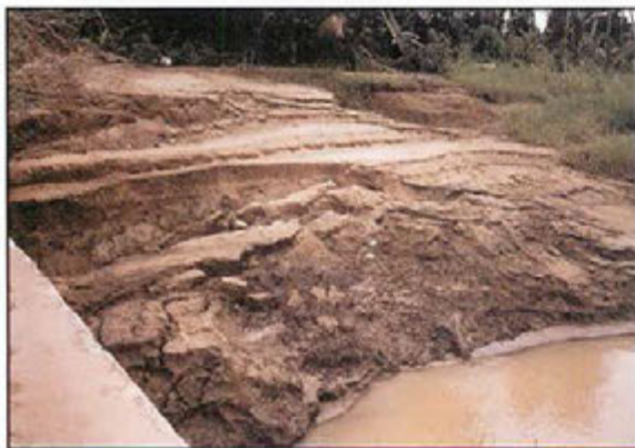
Fig. 11. Riverbank instability, Sarawak.
