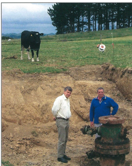
Indo-Pacific CEO with consultant and interested spectators at the Cheal 1 and 2 wellsite before the drilling rig arrived.
