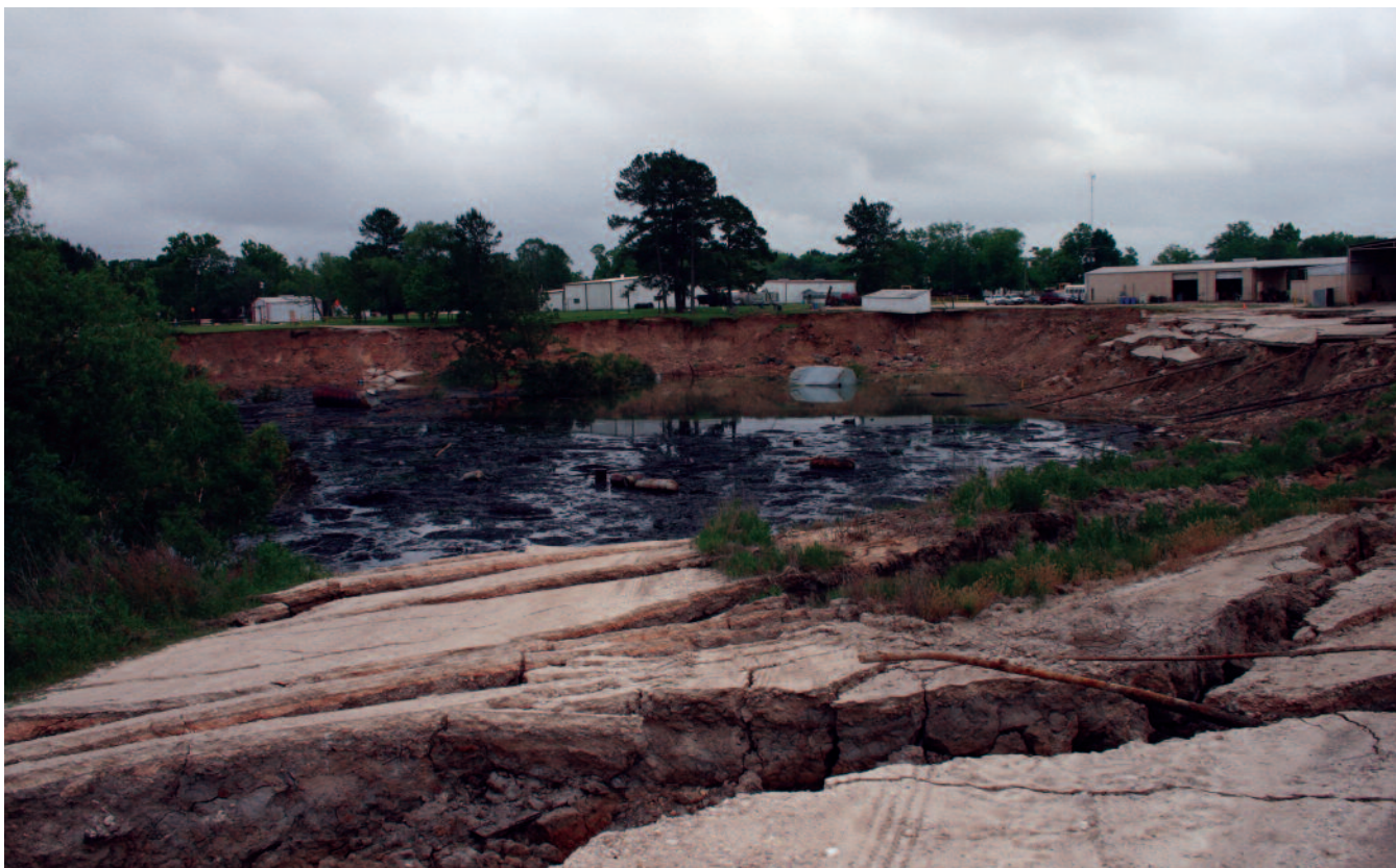
View southeast across the southern portion of the Daisetta sinkhole.
