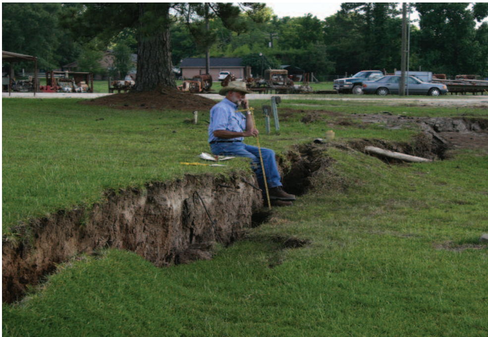
This photo is looking to the south-southeast across the crown, main scarp, and head of a slump block located along the southeast quadrant of the sinkhole. Dr. Carl Norman is sitting on the crown of the slump with his legs dangling across the block's main scarp and his feet hanging a few inches above the head of the slump.
