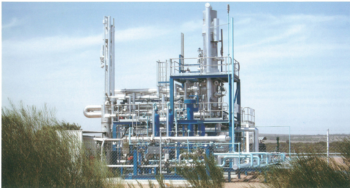
Cool Energy's CryoCell® plant in Dongara, Western Australia
