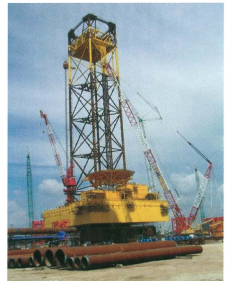
Near complete Maari wellhead platform in Lumut, Malaysia, awaiting loadout to New Zealand
