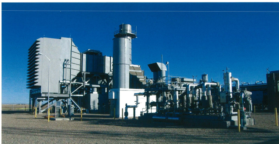
A General Electric 100 MW LMS100 gas-fired peaking unit
